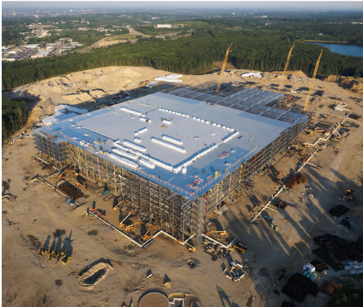
FOR MORE INFO: Visit New England Aerial Services' website at www.newenglandaerialservices.com . Visit their Facebook page at www.facebook.com/newenglandaerialservices . For a full gallery of more than a dozen aerial images from the Johnston Amazon construction site, go to the Johnston Sun Rise's website, www.johnstonsunrise.net . (Photos courtesy New England Aerial Services)
